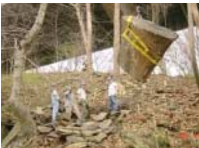
In the shadow of GW parkway, the crew pulls another boulder into place.
